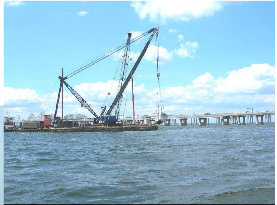
Photos by MDE Emergency Response Division
